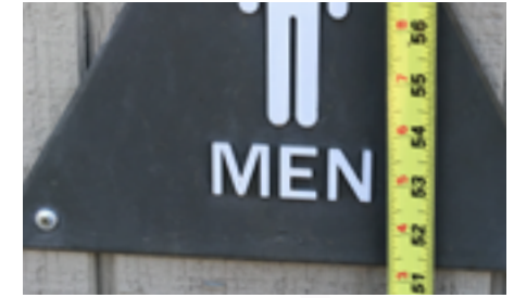
Center of Geometric signage too low.
