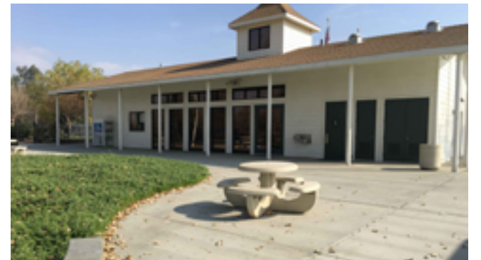
Circular benches do not accommodate wheelchair users.
