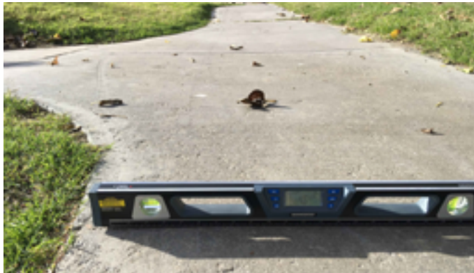
Typical example of excessive cross slope and running slope at walkway intersections.
