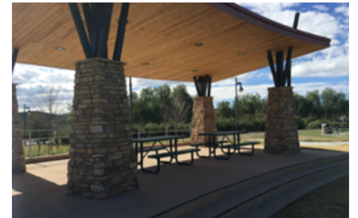
Stairs at amphitheater picnic shelter are absent of handrails.
