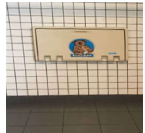
Baby Changing Stations cannot be located within Designated Accessible Toilet Compartments.
