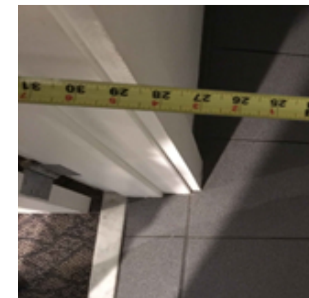
Toilet compartment entrance is only 28" wide.
