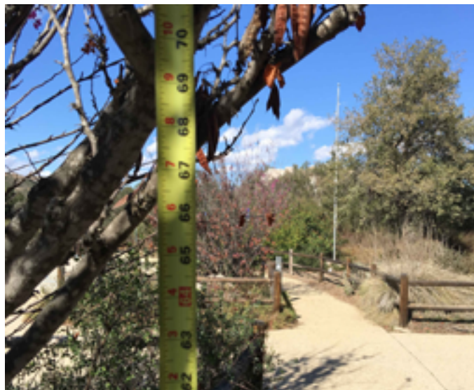
Low tree branches within walkway areas present overhead clearance issues. 80" minimum is required.
