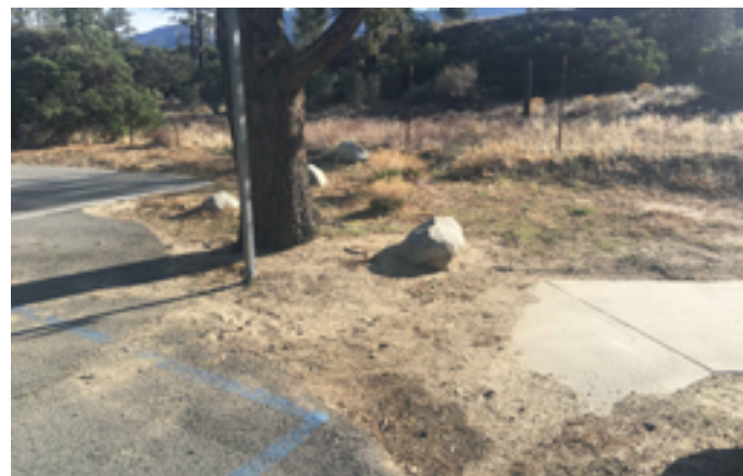
Excessive slope, debris on walkway surfaces, and subsiding asphalt all hinder the accessibility of the playground-adjacent parking.
