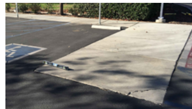
Replace uneven concrete, address paving gaps, and provide truncated domes where the walkway meets parking at a zero-curb condition.
