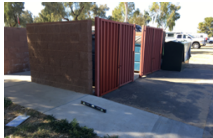
Access to trash enclosures exceeds allowable slopes, does not offer edge protection, and leads park patrons directly into hazardous vehicle area without detectable warning..
