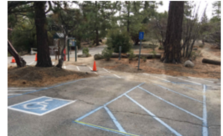
Parking area near park entry. Access aisle measured approximately 3" narrower than the required 8' width.
