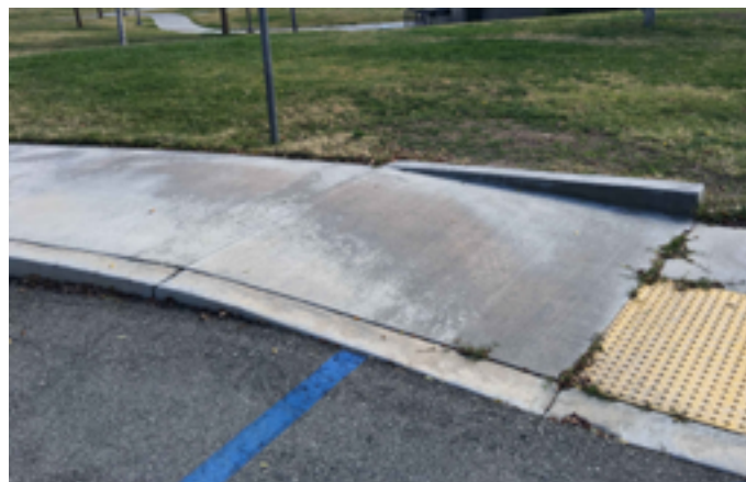
Asphalt near the zero-curb/ detectable warning area is built up, causing slope to exceed the 1:48 maximum within the loading zone of this parking space near the Splash Pad.
