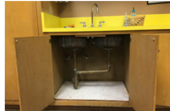
No knee/ forward wheelchair approach at sink.
