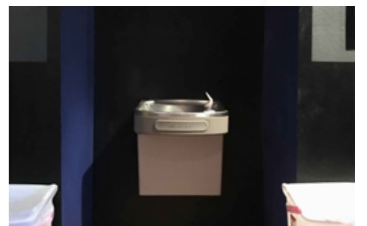
Drinking fountain missing its 2nd fountain companion.
