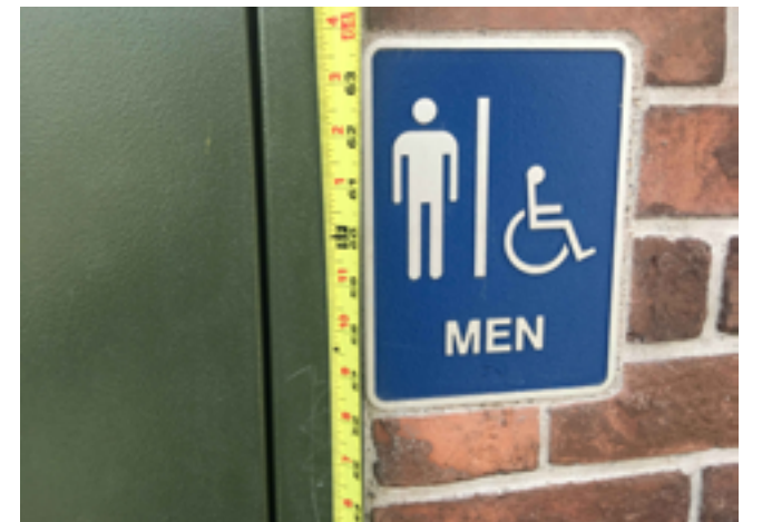
Pictogram signage at proper location.
