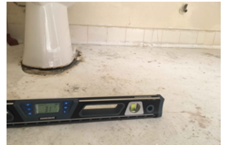
Excessive slope at restroom floor.
