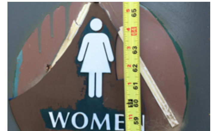
Women's room geometric sign is damaged.
