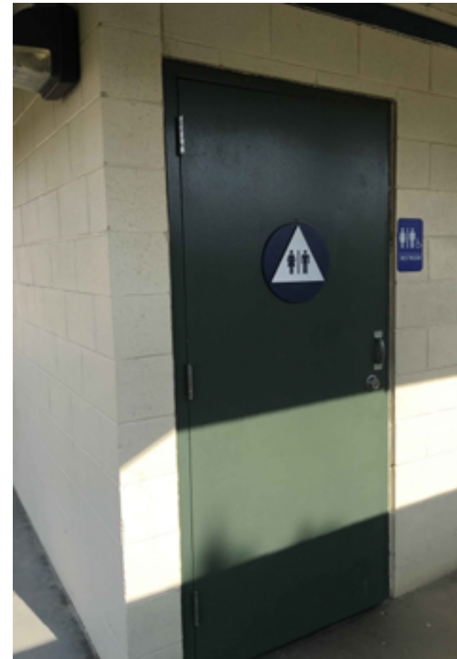
Geometric signage at proper height.
