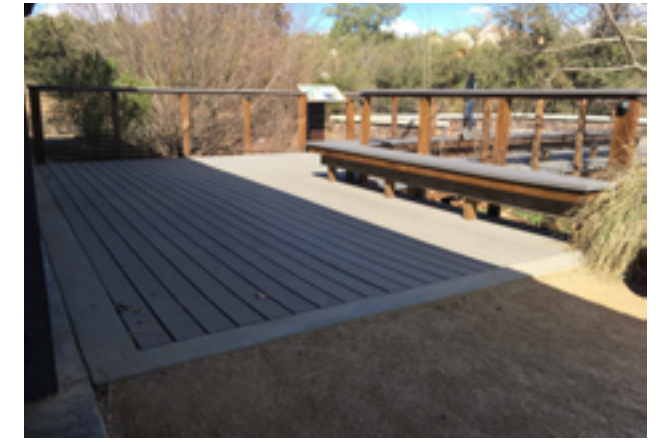
Integral benches at the boardwalk measure approximately 18" in depth, which does not meet the minimum required depth of 20".
