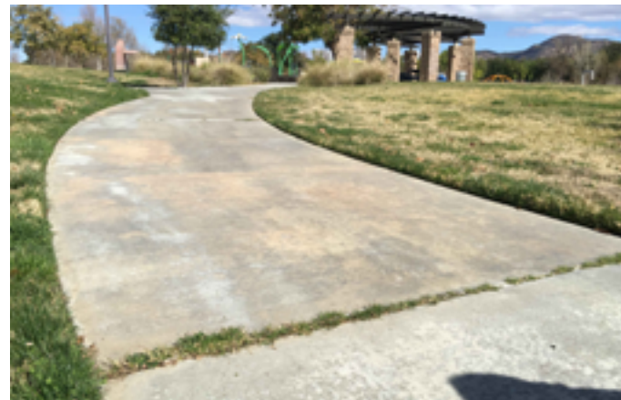
Another view of non-compliant sloped walkway. Also, some joints appear to exceed gap tolerances, but gaps are currently being filled with lawn.
