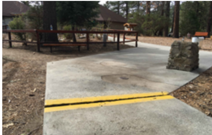
Yellow paint serves as a temporary warning of the vertical rise at the walkway joint. Note: the historic drinking fountain pictured is supplemented with an accessible high-low fountain (not pictured).
