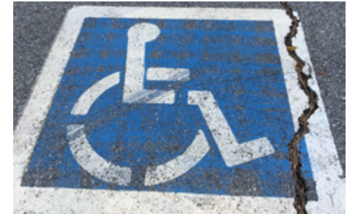
Large crack present within existing DAPS.
