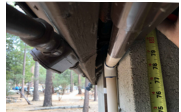
Overhead obstruction at restroom entry.
