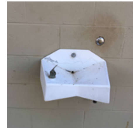
Non-compliant drinking fountain.
