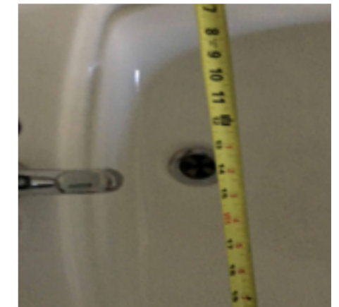
Sink too close to wall.
