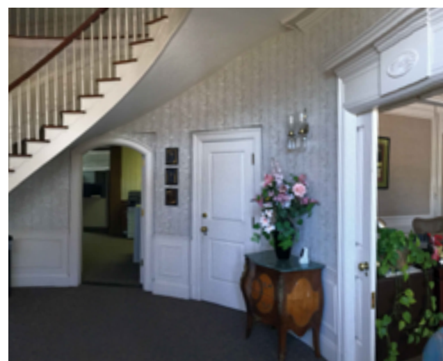
The underside of the curved portion of the staircase, as well as the arched doorway beneath, provide vertical obstructions without cane detection warning.
