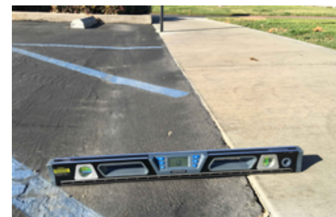
Example of excessive slope observed within the passenger loading zone between DAPS #1 and 2;
