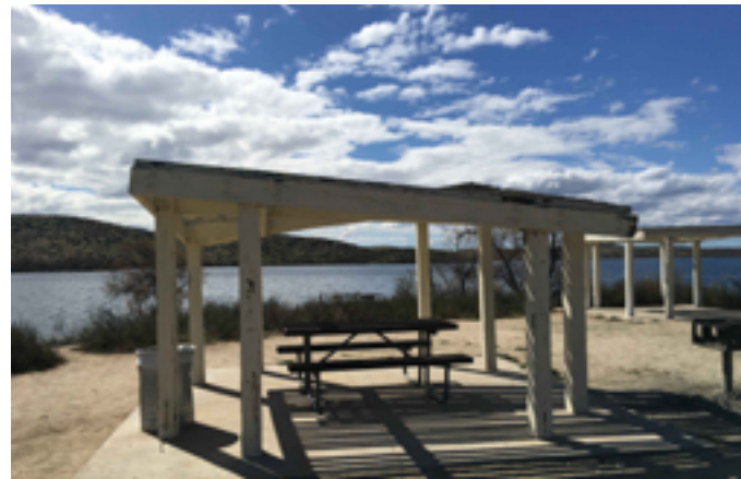
Many shelters have beams as low as 63" above finish grade, and would need to be removed and replaced to eliminate vertical clearance issues.
