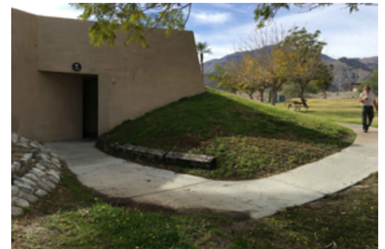
Non-accessible walks leading to restroom.
