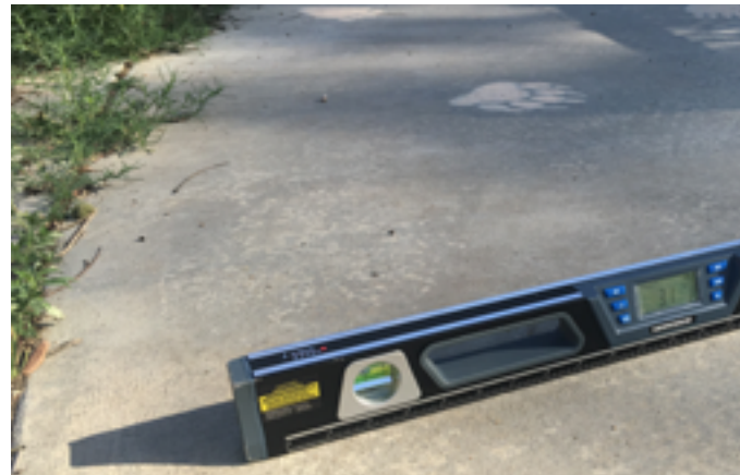
Excessive cross slope is noted on the walkway between the parking area and the Nature Center building.
