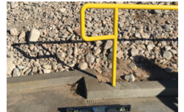
The access ramp continues to ascend past the handrail extension.
