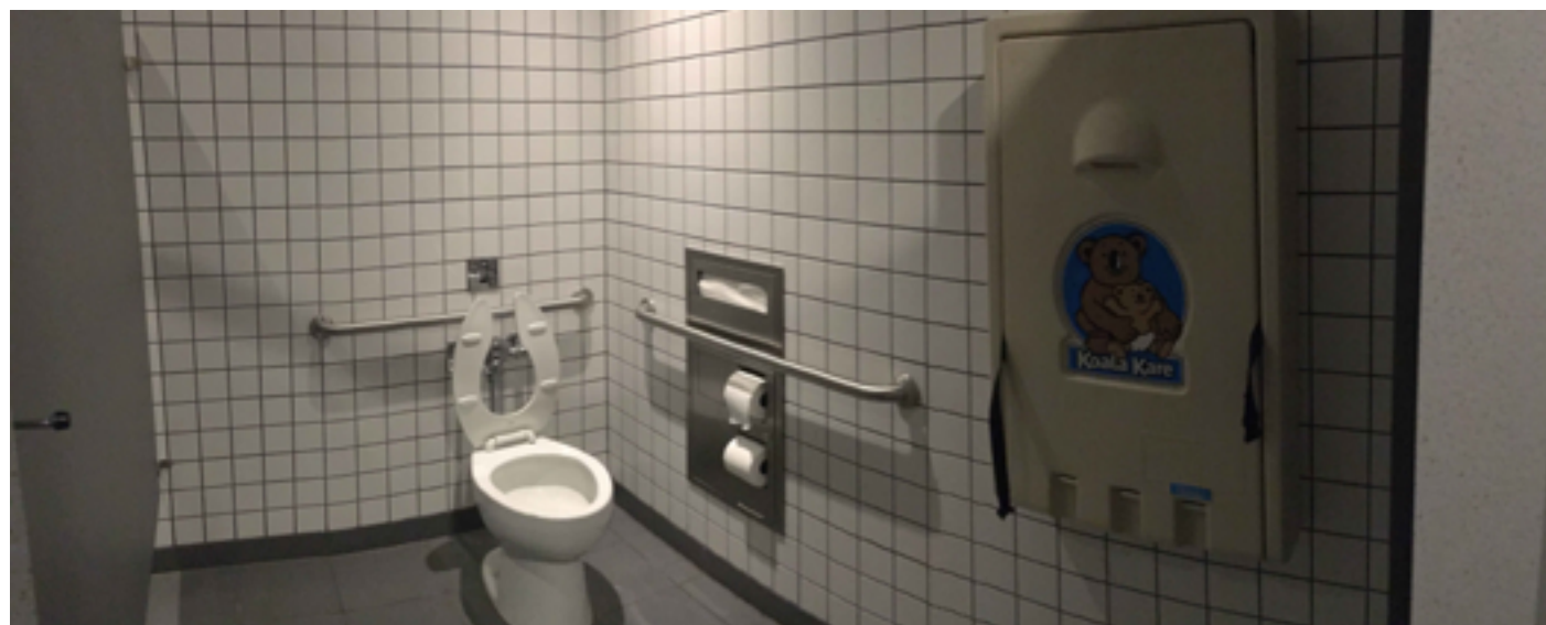
Overview of Women's Room Accessible Toilet Compartment. The Baby Changing Station will need to be relocated out of Accessible Toilet Compartment.
