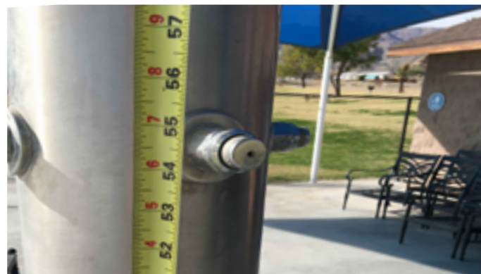
Shower actuation buttons are located outside of reach range for wheelchair users.
