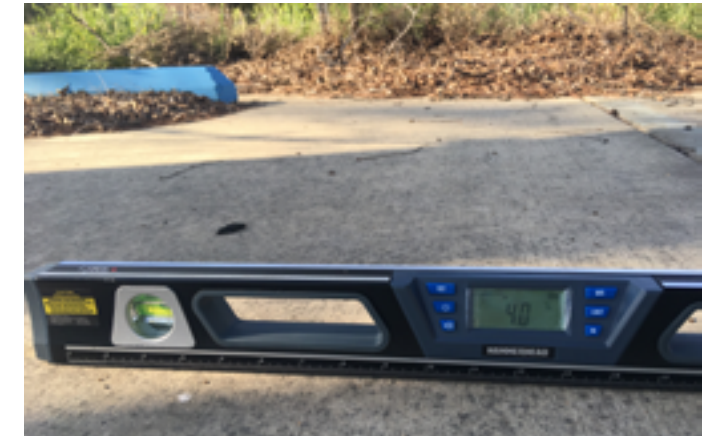
All Designated Accessible Parking Spaces and Access Aisles exceeded the 1:48 (2.08%) slope. Pictured above: 4% cross slope.
