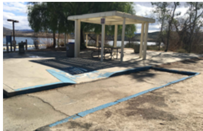
This non-compliant curb ramp leads wheelchair users directly to and from a hazardous vehicle zone.
