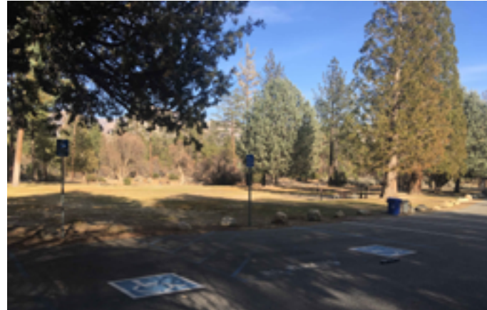
Parking at the south edge of the Meadow area is missing "Van Accessible" and "MINIMUM FINE $250" signage; Loading zone does not connect with any accessible site features nor buildings.
