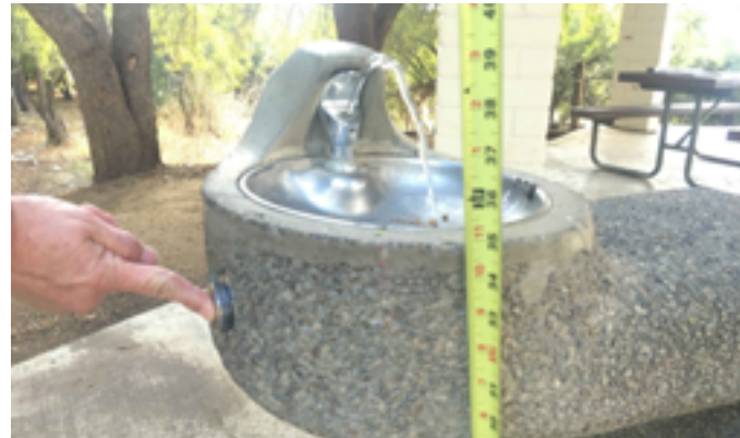
The drinking fountain does not meet the height requirements for either of the two height ranges: wheelchair accessible spout at 36" max, or standing person spout outlet between 38"-43".
