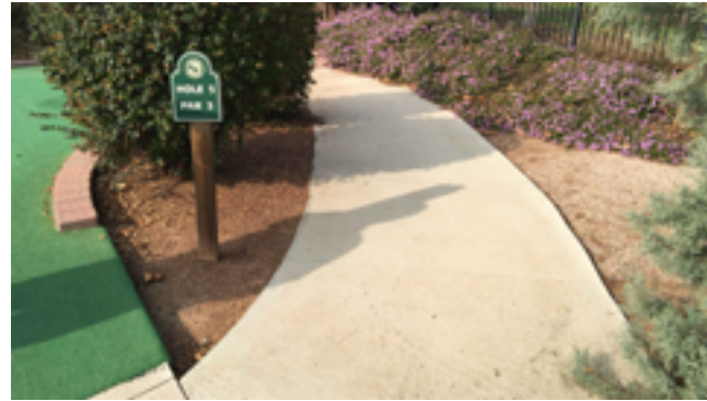
Hole 5 bypass walkway exceeds maximum allowable running slope for walks, and should be reconstructed as a ramp.
