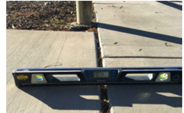
Large gaps were present at concrete joints.
