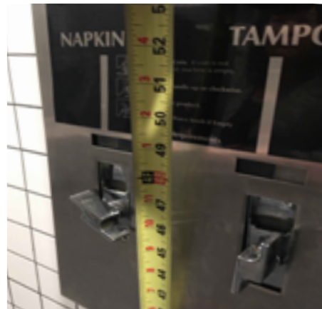
Operable parts of dispenser exceed 40" maximum AFF.
