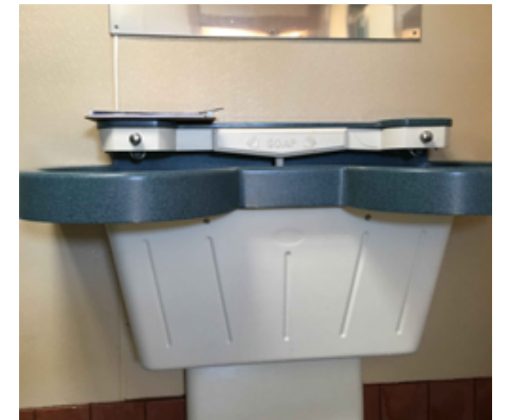
Non-standard, non-accessible sink within restrooms.
