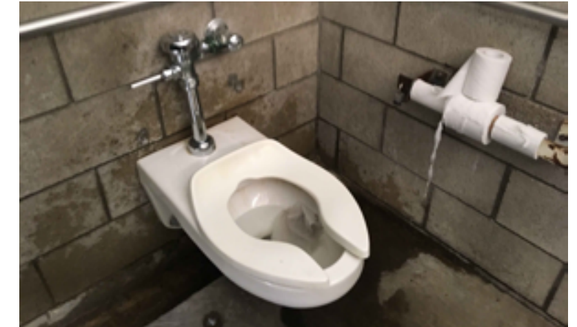
Floor drain trough does not meet accessibility standards.
