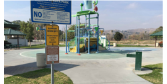
Signage overhangs above the walkway edge at 78" as measured in field. 80" min. clearance is required.
