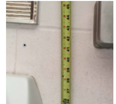
Men's room soap dispenser and mirror mounted too high.
