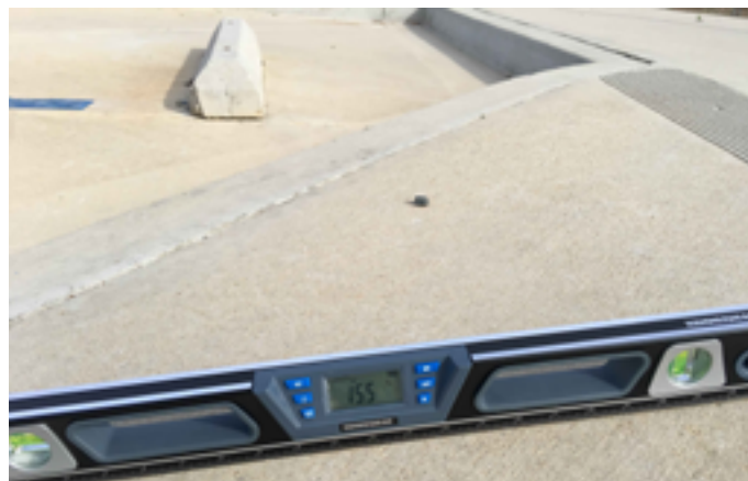
Example of excessive slope observed at the curb ramp.
