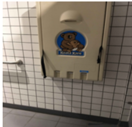
Baby Changing Stations cannot be located within Designated Accessible Toilet Compartments.
