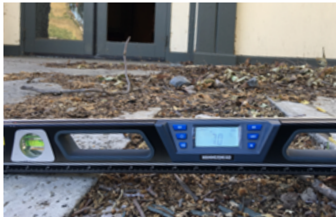
Excessive slope, vertical changes in level, and scattered debris is present throughout the concrete plaza and walkways surrounding the Nature Center building.
