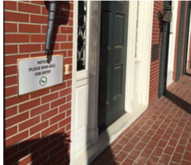
Access to the Front Door of the Manor House is impeded by a pronounced threshold. However, this door is not currently used as a primary entrance point into the building.
