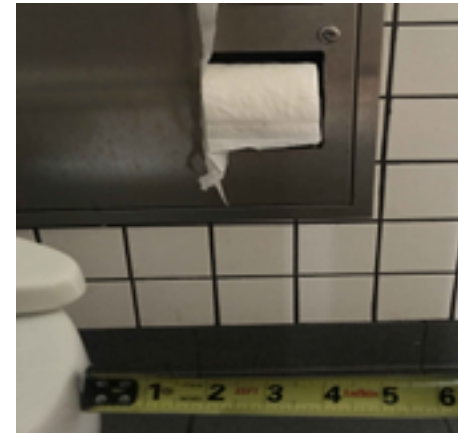
Centerline of Toilet Paper is required to be between 7" and 9" in front of toilet. Current location is approximately 3" in front of toilet.
