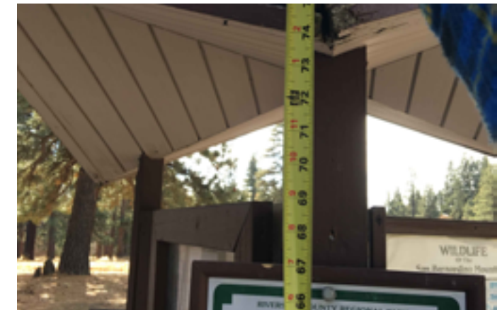
This information kiosk has three eaves that cause vertical clearance obstructions at approximately 74" above finish grade.
