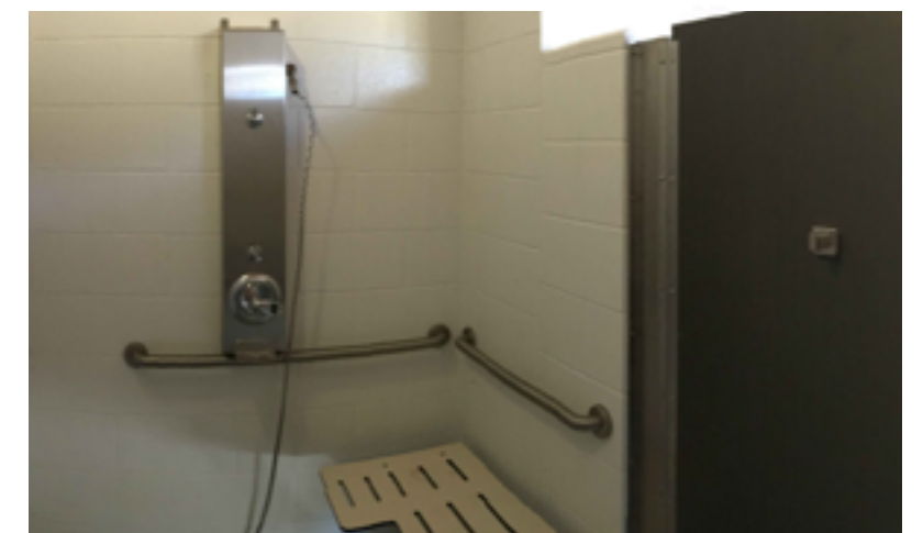
Grab bar above improperly mounted shower seat.
