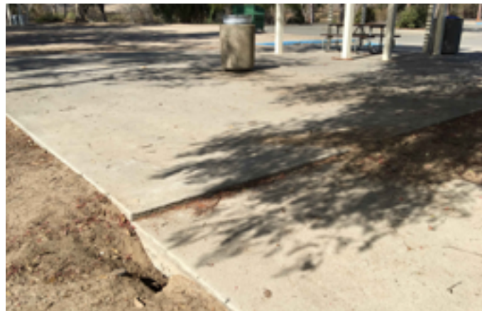
Walk surfaces include major vertical "steps" requiring removal and replacement.
