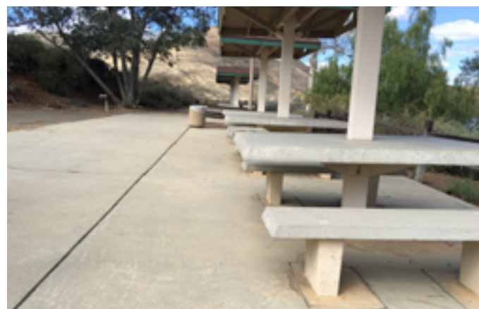
The entire area contains excessive running and cross slopes.
