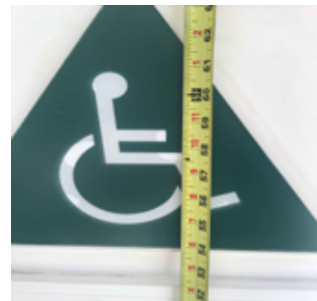
Center of geometric sign is required to be 60" AFF. Sign is currently 57" to 58".
