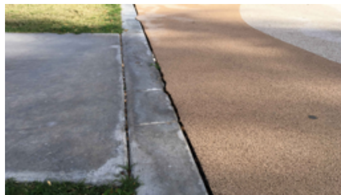
Playground surfacing is separating from perimeter curb, creating a gap larger than the maximum 1/2" allowable by accessibility codes.
