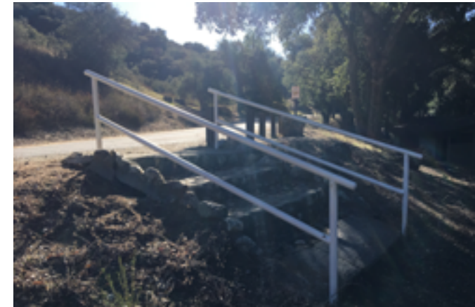
These stairs would require a complete renovation to meet accessibility standards.
