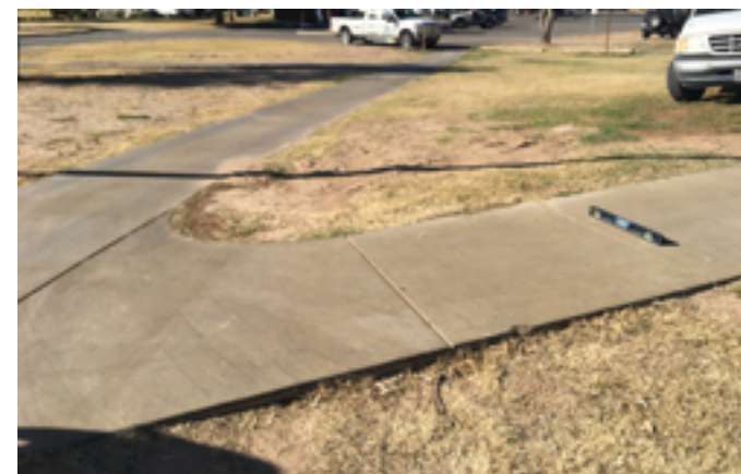
The walkway accessing the new restroom/ shower building exceeds allowable cross slope, at and near wheelchair turning space.
