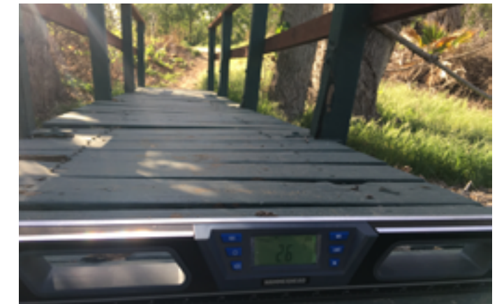
Excessive cross slope is noted on the bridge.
