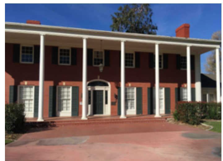
Handrails are not present anywhere along the two-step level change leading to the front door.
