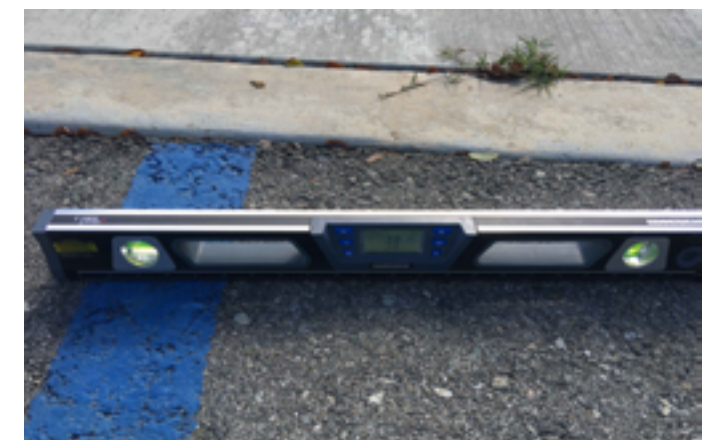
Example of excessive slope observed within the passenger loading zone near the Splash Pad;
