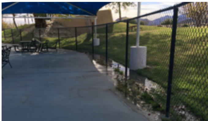
Non-recreational standing water is present within the circulation area.
