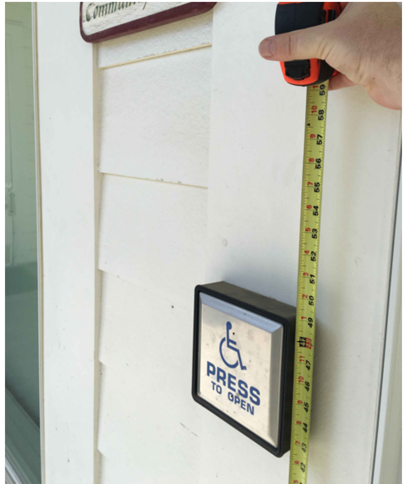
Press to continue. (This image shows a functional automatic door activation button within proper reach range; no corrections necessary)
