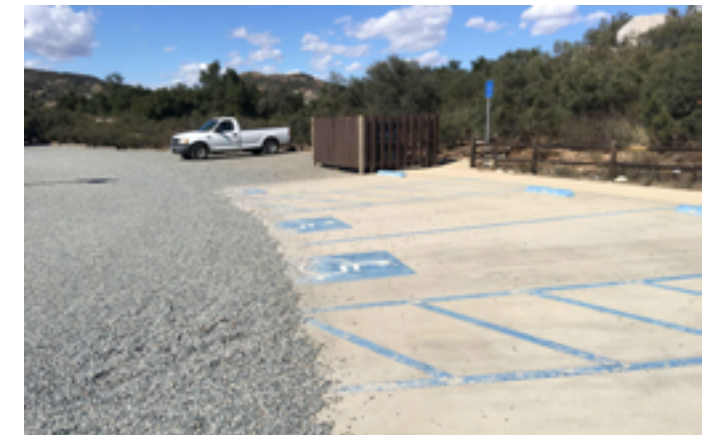
Gravel, worn striping, lack of No Parking paint.
