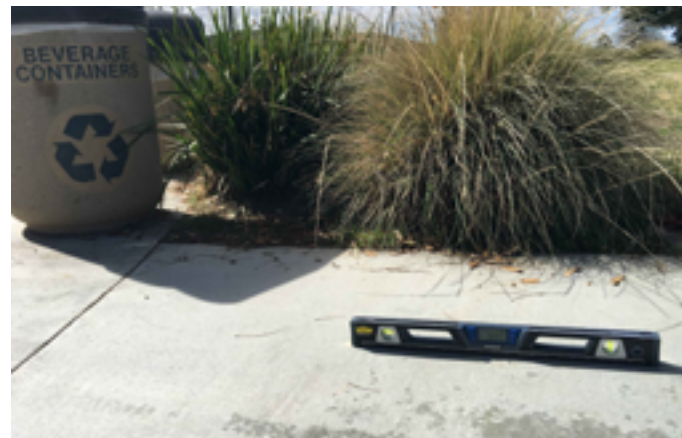
Portions of the pedestrian route exceed 1:20 without the presence of handrails nor landings. Adjacent path intersections also exceed maximum slope for wheelchair turning.
