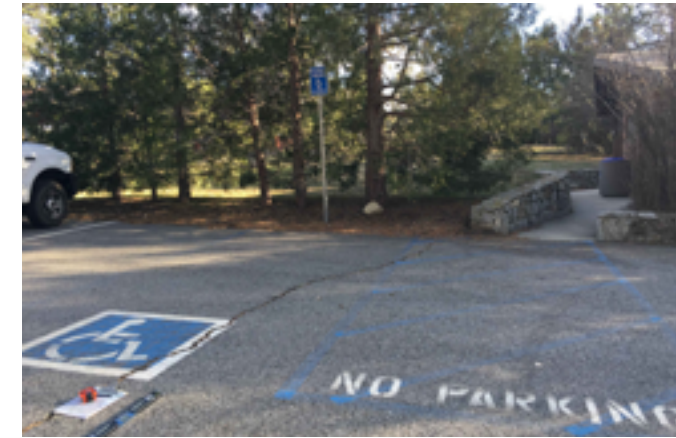
Designated Accessible Parking Space has excessive slope, faded striping, surface issues, and missing "MINIMUM FINE $250" signage.
