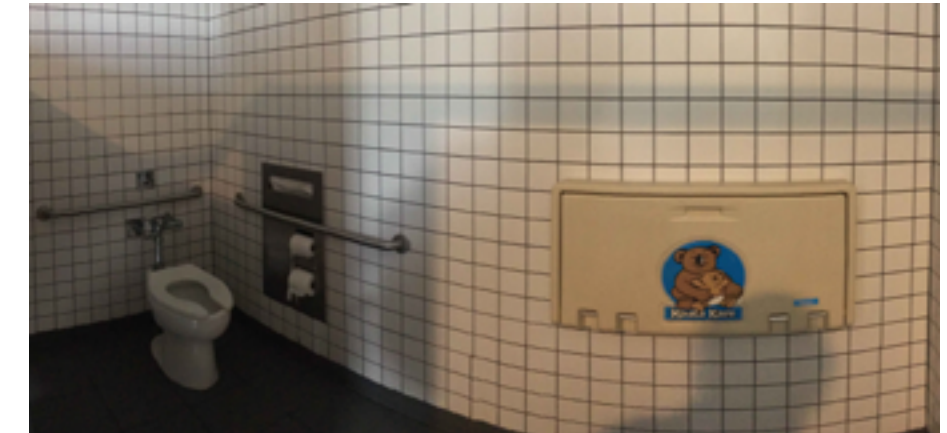
Overview of Men's Room Accessible Toilet Compartment; need to remove baby changing from toilet compartment.
