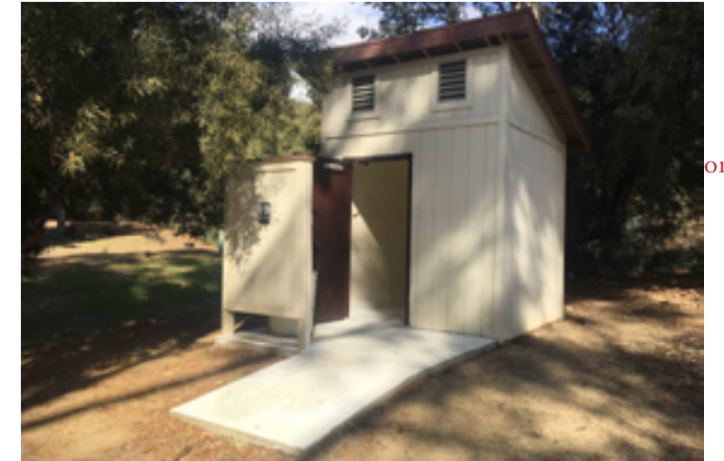
Excessive slope to restroom entry.
