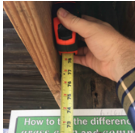
Low beam height at one shelter, as noted in Action Item 2.6.4
