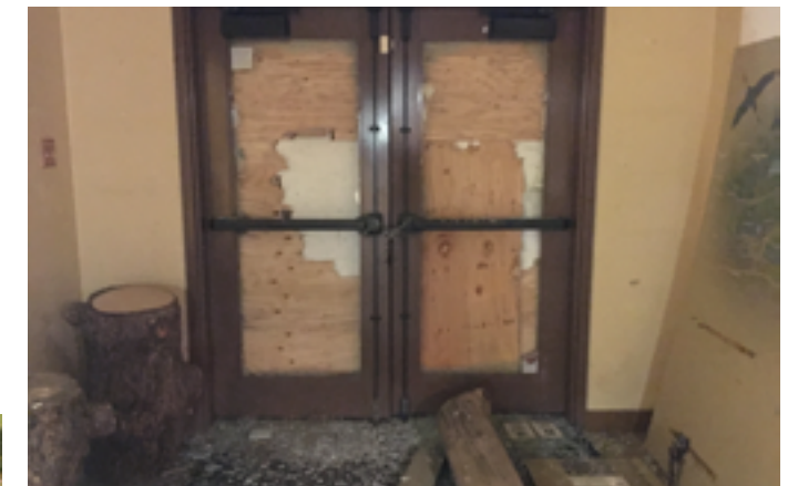
Insufficient kick plate height at exit doors.
