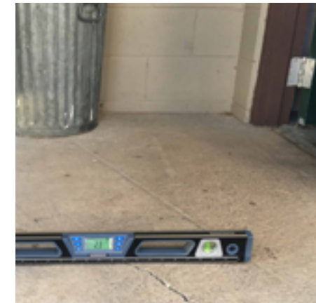
Excessive slope at restroom entry.
