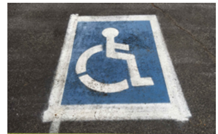
Example of improper proportions of International Symbol of Accessibility (ISA)
