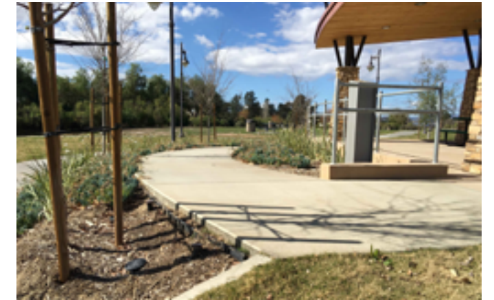
Edge protection is needed at walkway leading up to amphitheater picnic shelter.
