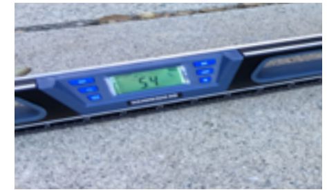
Excessive slope in perimeter concrete slabs.
