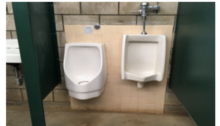
The absence of a splash guard/modesty partition between urinals allows for forward wheelchair approach.
