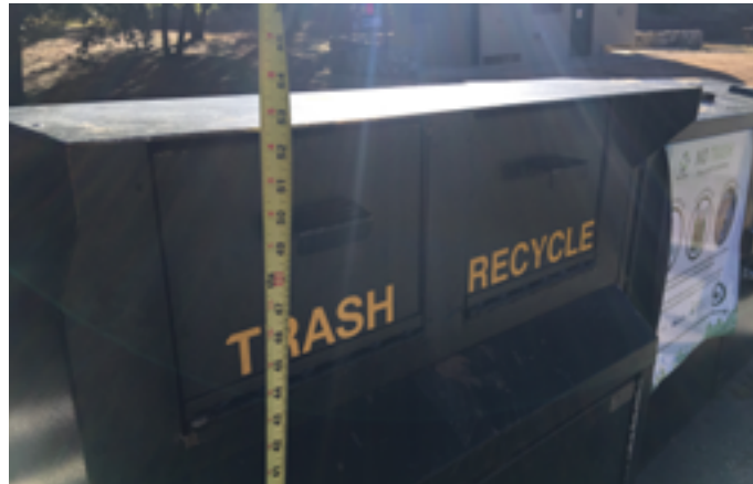
Both of the waste and recycling receptacles require movements above the maximum reach range for operable parts of 48" maximum as defined in CBC 11B-308.3.1 (see Unobstructed Side Reach)
