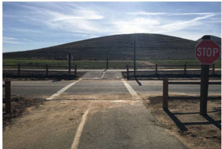
Pedestrian crossing surface has been compromised by soil runoff at Hidden Valley Nature Preserve.
